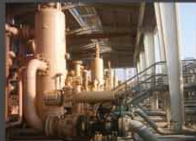
SAJGAS Plant - UAE
