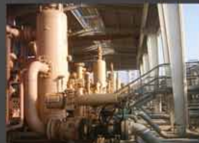
SAJGAS Plant - UAE
