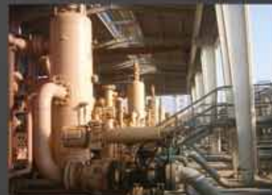
SAJGAS Plant - UAE
